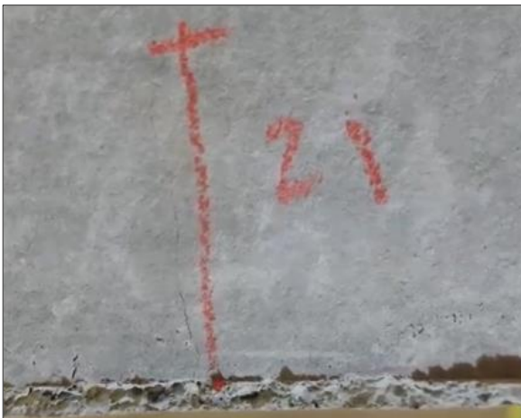
Fig 7.6. First crack as observed
